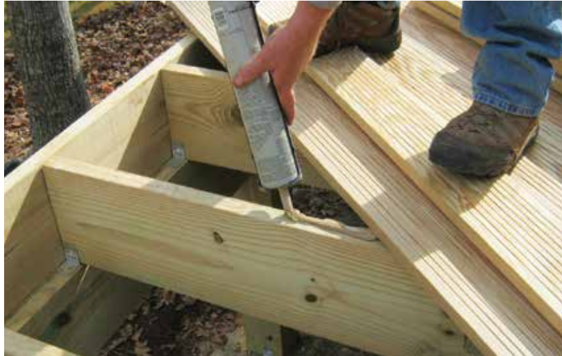
Figure 5. To provide a stronger connection, the author often uses construction adhesive when installing T&G or shi lap porch flooring.
